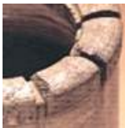
LOSS OF INSIDE DIAMETER
